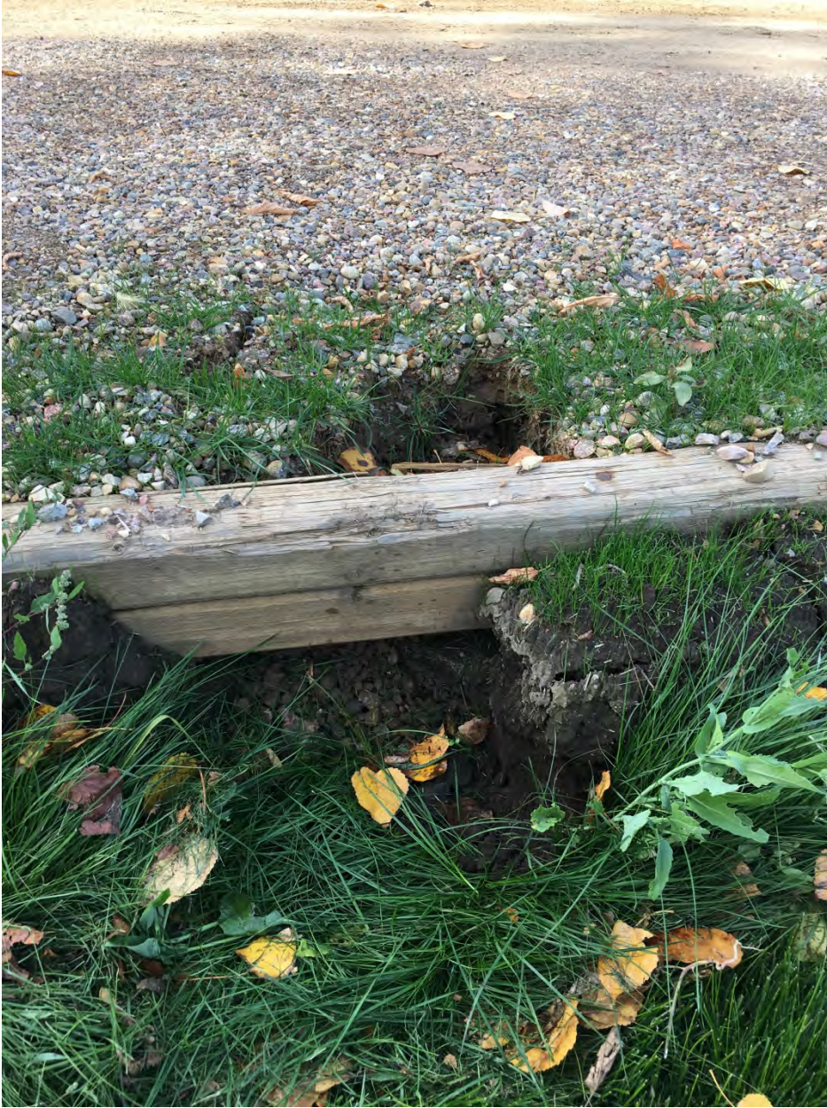
10010 and 10014 Access culvert. Will be repaired shortly.
