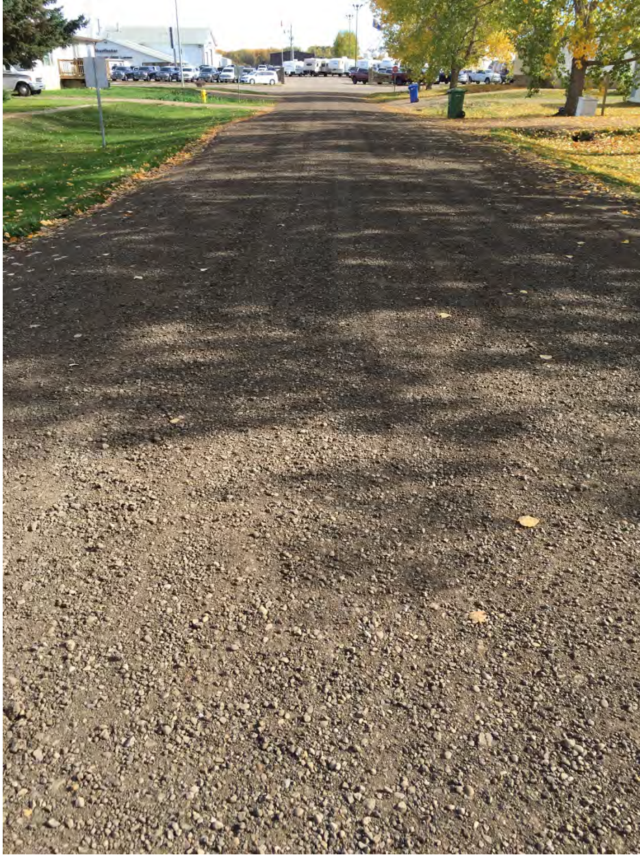
Asphalt Millings by 10014-96 Avenue
